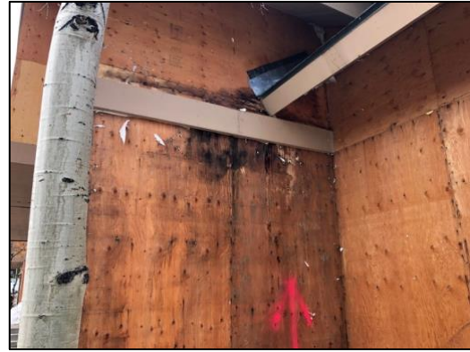
Bldg E4 Unit #28 Entry Exterior Mold - 1
