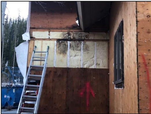
Bldg E4 Unit #28 Entry Exterior Mold - 2
