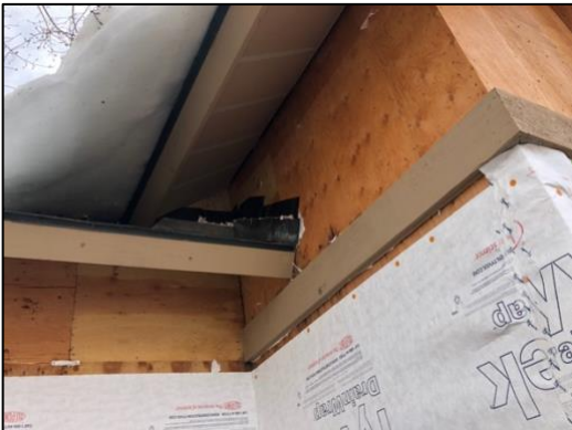
Existing Step Flashing In Place – No Diverter
