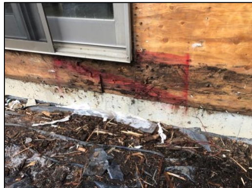
Bldg E1 Unit #9 Deteriorated Lumber
