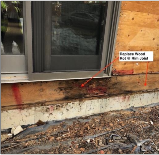
Bldg E1 Unit #8 Rotted Rim Joist
