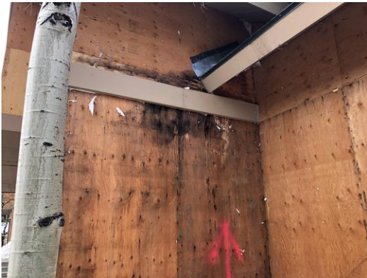
Bldg E4 Unit #28 Discoloring
