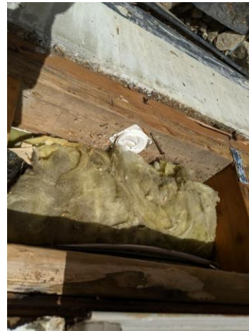
Building E4 Unit #28 Possible Pest Control Problems
