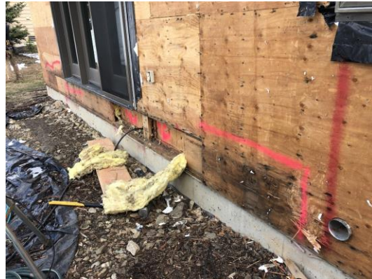
Bldg E4 Unit #28 Discoloring
