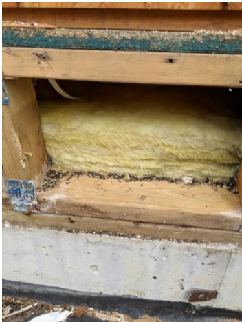
Building E4 Unit #21 Possible Pest Control Problems
