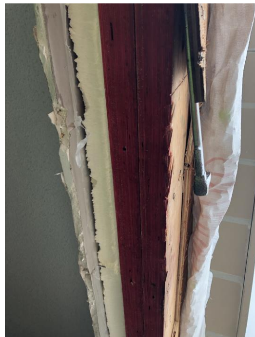
Bldg E3 Units #25 Window Head Exposed
