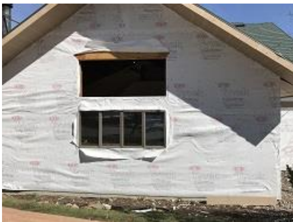
Bldg E4 Unit #31 Upper Window
