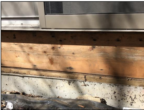
Bldg E1 Unit #10 Wood Member Exposed Horizontal Split
