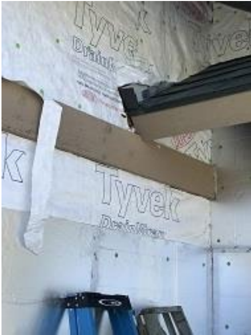
Building E1 Unit 11 Diverter Flashing
