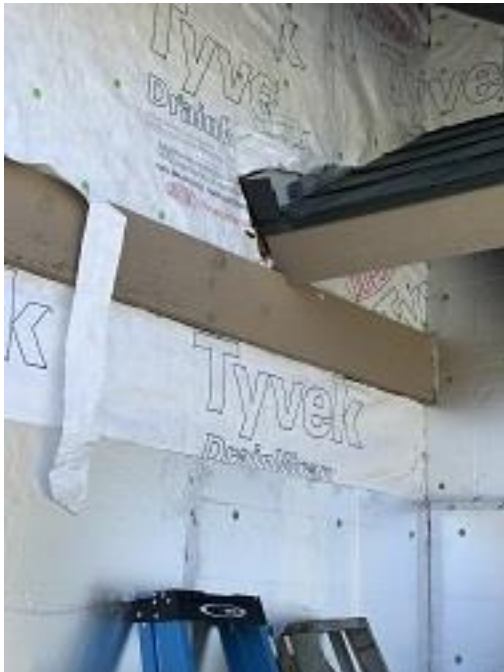
Building E1 Unit 11 Diverter Flashing
