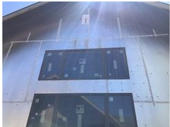
Building E3 Unit 24 Metal Flashing Missing
