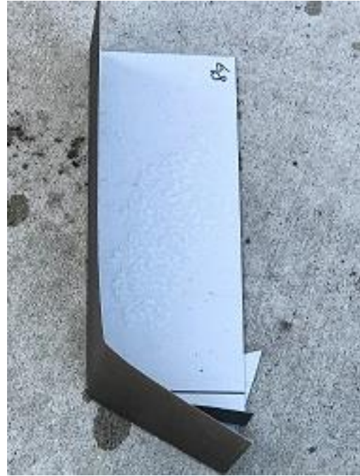
Building E1 Unit 11 Diverter Flashing
