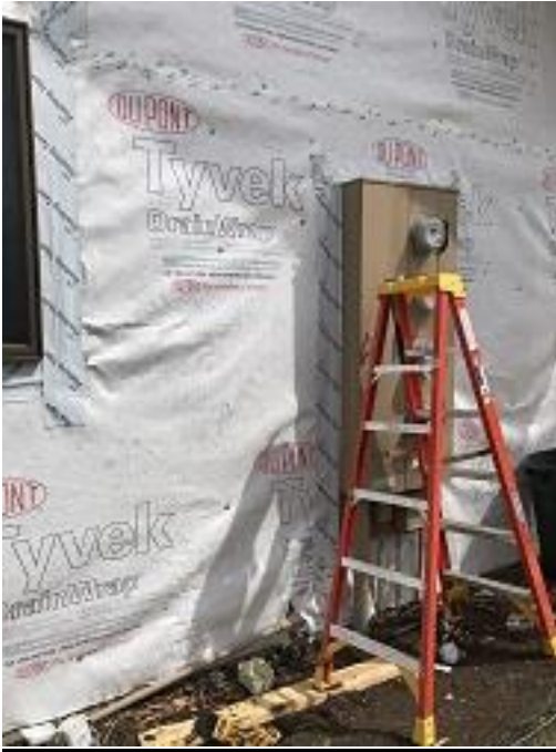
Bldg E2 Electrical Panel Flashing Tape
