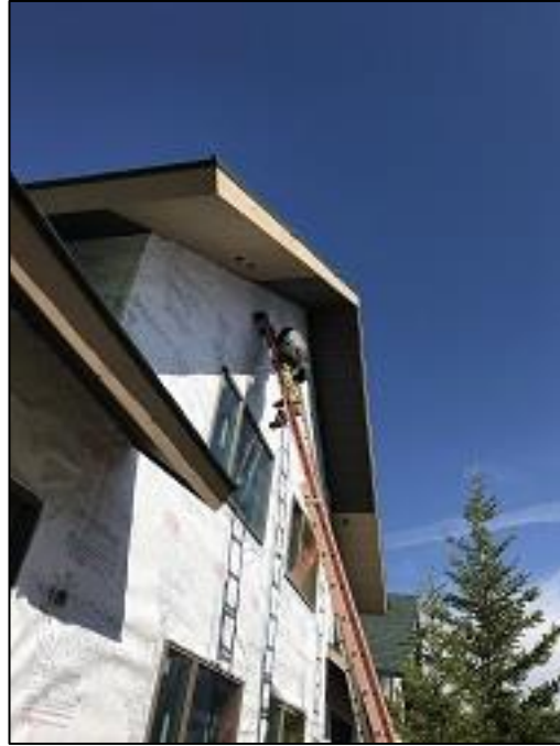
Bldg E3 Unit #26 & #27 Rear Gable Soffit
