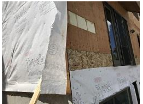
Bldg F1 Unit 16 Upper Deck Railing Blocking Location Cut Out
