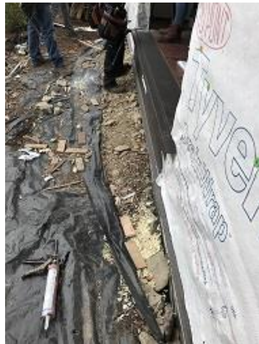
Building E3 Unit 24 Patio Door & Deck Ledger Flashing
