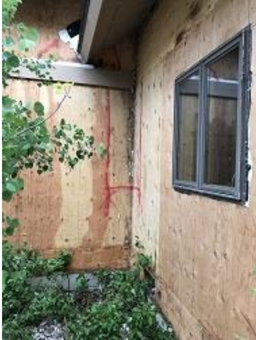
Building E7 Unit 49 Front Damage Area
