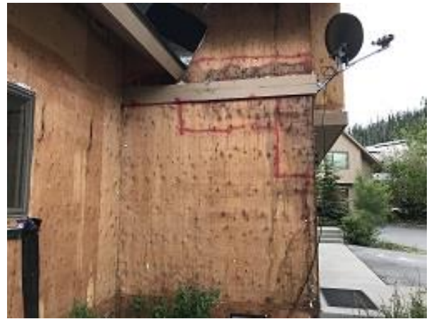
Building E7 Unit 50 Front Damage Area
