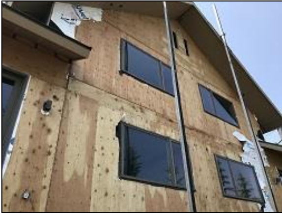
Building E7 Units #49 & #50 Gable Vent Cut Outs
