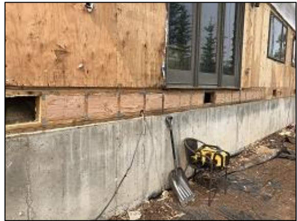
Building E7 Unit #49 Deck Ledger Blocking
