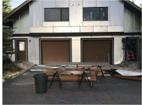
E3 Unit 26 & 27 Belly Band Steel Installed and Unit J Channel Around Garage Trim Installed
