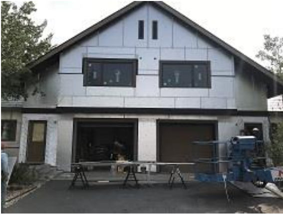
Belly Band Steel Installed and Unit 24 J Channel Around Garage Trim Installed
