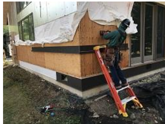
Building E4 Unit 28 Base and Wainscot Flashing, Deck Hand Rail Blocking Installed
