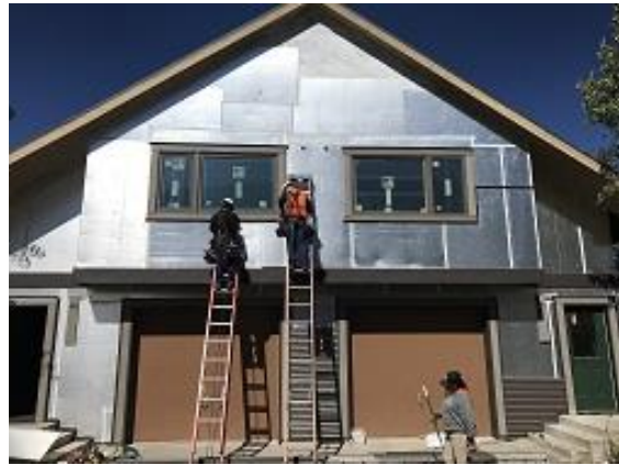
Building F1 Units 16 & 17 Front Window Trim, Foam Board and J Channel Installed
