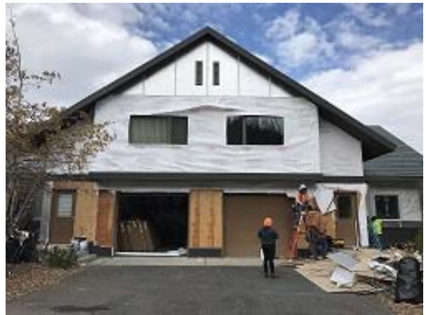
Building F2 Units 18 & 19 Front Tyvek, Belly Band, Base Flashing & Foam Board Install
