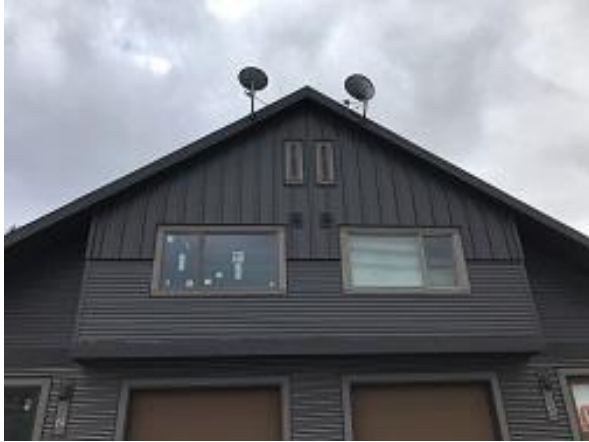
Building E1 Units 8 & 9 Satellite Dishes Installed
