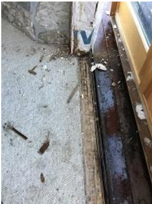
Building E7 Unit 52 Deck Door Threshold Damage
