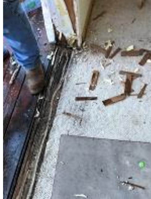
Building E7 Unit 52 Deck Door Threshold Damage
