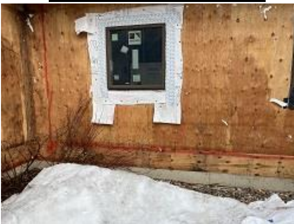
Building E8 Unit 57 Front Sheathing Removed with Moisture Higher Than 10%
