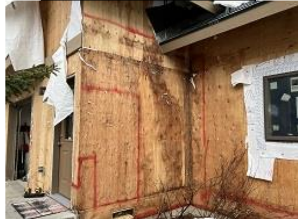
Building E8 Unit 57 Sheathing Removed with Moisture Higher Than 10%
