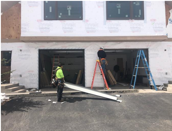
Building E8 Units 55 & 56 Garage Door Trim
