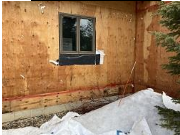
Building E8 Unit 56 Front Sheathing Removed with Moisture Higher Than 10%
