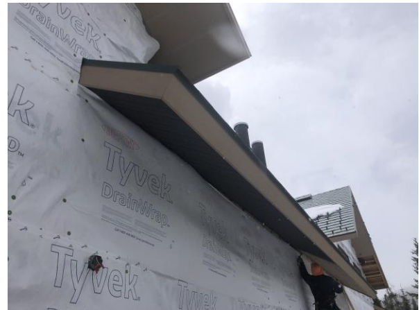
Building E8 Unit 56 & 57 Rear Soffit
