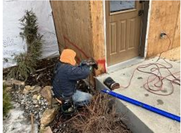
Building E8 Unit 58 Sheathing Removed with Moisture Higher Than 10%
