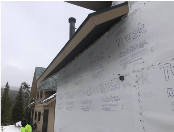
Building E8 Unit 55 Rear Soffit
