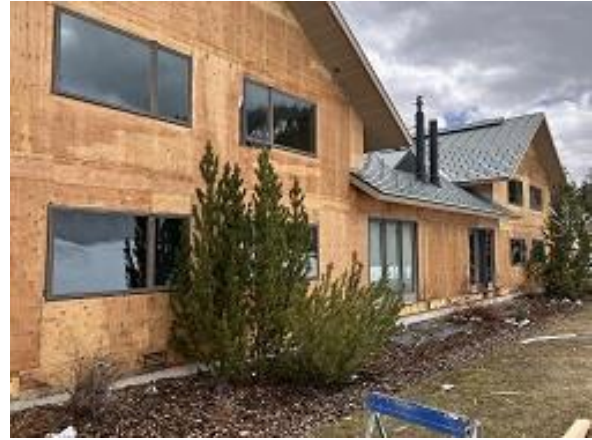
Building E6 Unit 47 & 48 Back Sheathing Exposed
