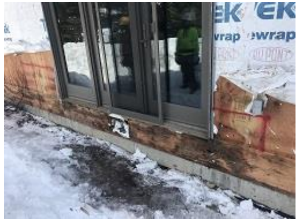
Building E8 Unit 57 Back Door Area Moisture Level Above 10%
