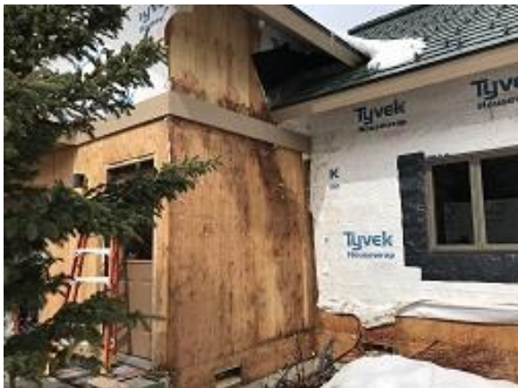
Building E8 Unit 57 Front Sheathing Exposed Moisture Level Above 10%
