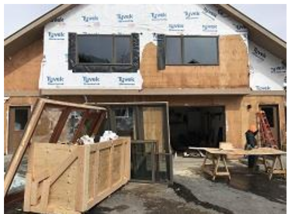
Building E8 Unit 57 & 58 Front Sheathing Exposed Moisture Level Above 10%
