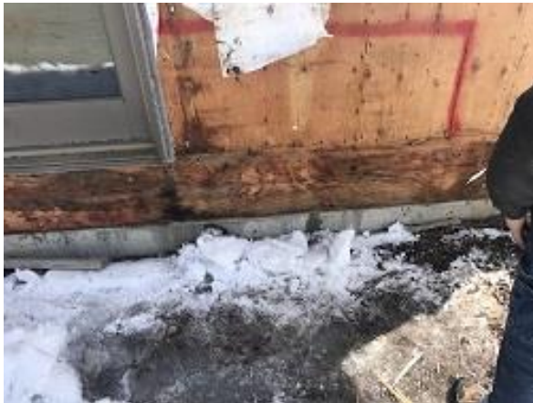
Building E8 Unit 58 Back Door Area Moisture Level Above 10%
