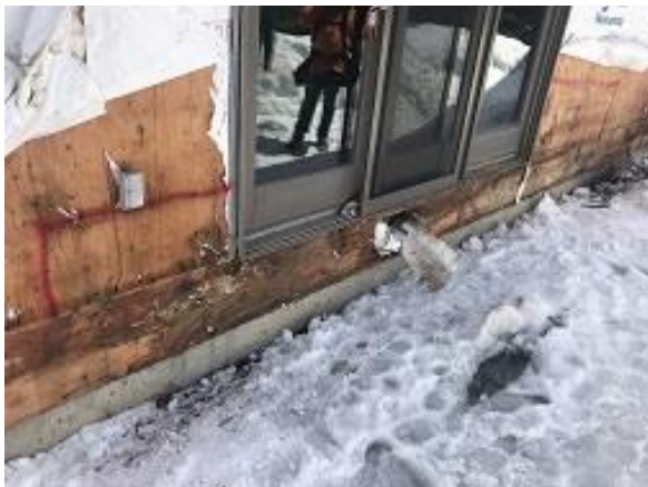
Building E8 Unit 56 Back Door Area Moisture Level Above 10%
