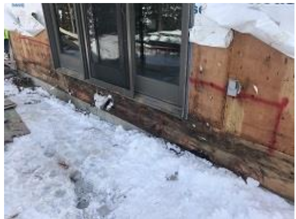
Building E8 Unit 55 Back Door Area Moisture Level Above 10%
