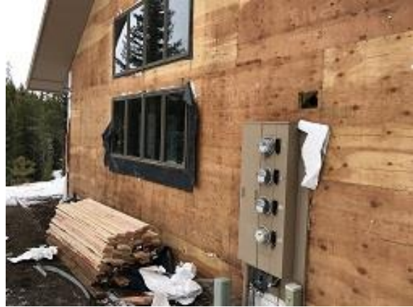
Building E8 Unit 58 Side Sheathing Exposed Moisture Level Below 10%
