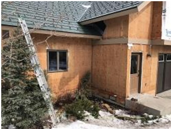
Building E8 Unit 58 Front Sheathing Exposed Moisture Level Below 10%
