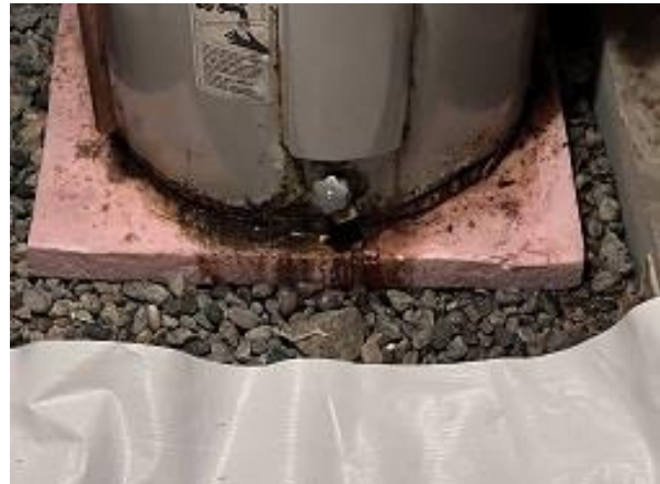
Building E6D Unit 45 Water Heater Leaking
