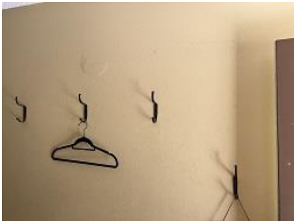
Building C1 Unit 12 Front Substrate Repair Caused Interior Damage
