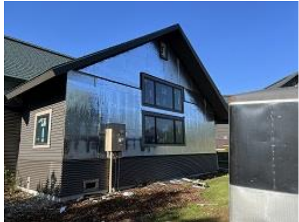
Building C5 Units 40 Snap Batten Flashing, Insulation, Window Trim & J Channel Installed
