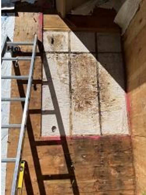
Building C1 Unit 12 Front Substrate Damage
