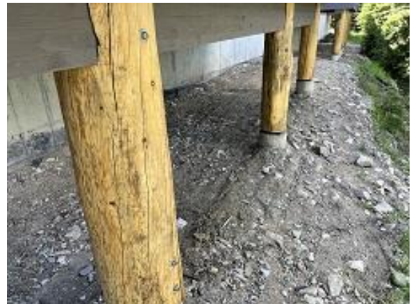
Building E7 Units 49 - 51 Deck Posts Stained
