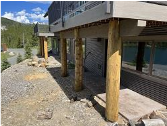
Building F2 Units 18 & 19 Deck Posts Stained
