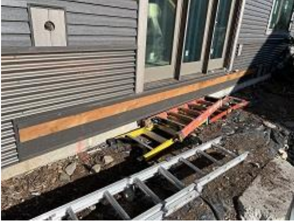
Building E5 Units 41 - 44 Deck Ledger Board 2x8 Wrong Size Should Be 2x10
