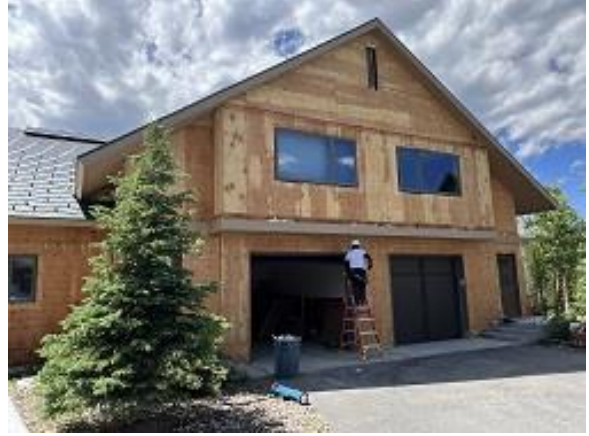
Building C7 Units 59 & 60 Front Sheathing Exposed
