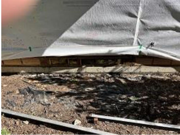
Building C2 Unit 15 Deck Ledger Mold Treatment
