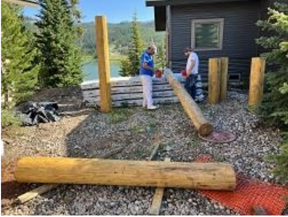
Building E7 Unit 52 & Building E5 Unit 44 Deck Posts Stained
