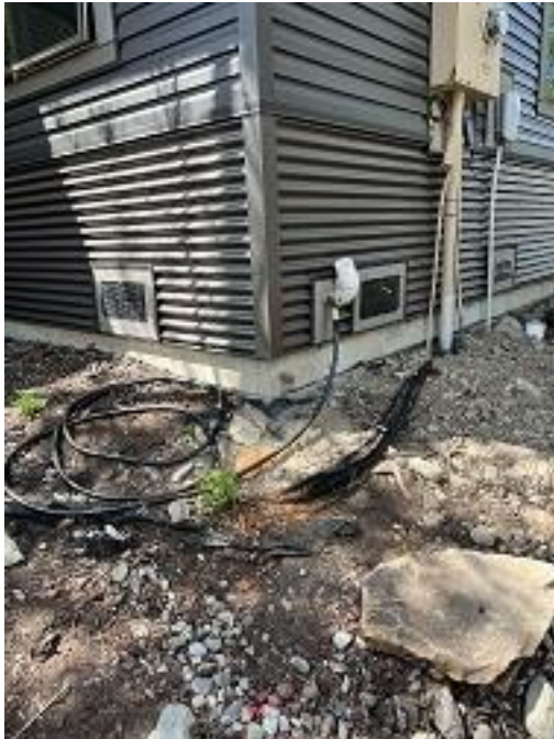
Building F2 Unit 16 Side Radon System Exhaust
