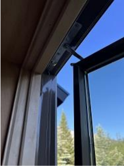
Building E8 Unit 56 Back Lower Window Rivet Broken
