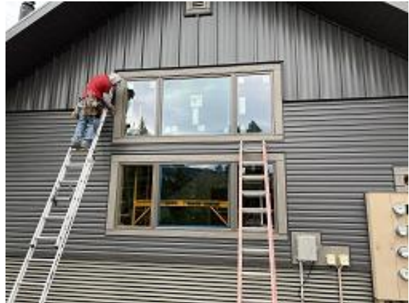
Building E8 Unit 58 Side Window Moved to Correct Location in Rough Opening
