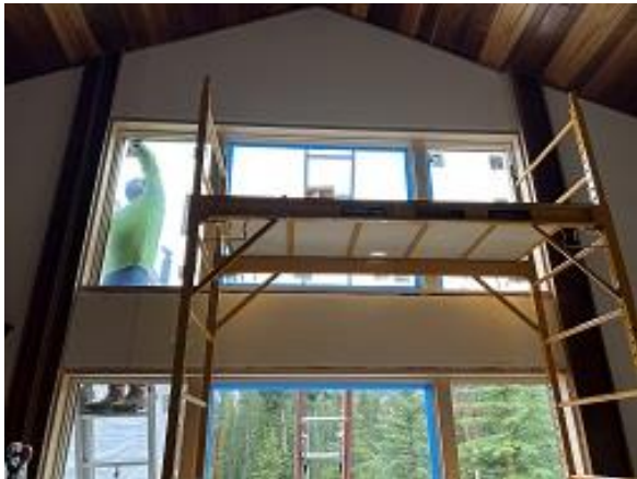
Building E8 Unit 58 Side Window Moved to Correct Location in Rough Opening
