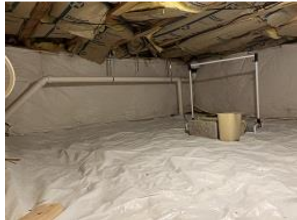
Building F2 Unit 16 Radon System Installed
