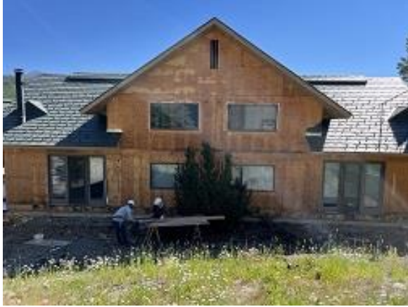
Building C9 Units 67 & 68 Back Sheathing Exposed
