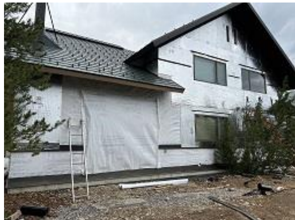
Building C3 Units 32 & 33 Back Head & Snap Batten Flashing and Insulation Board Installed
