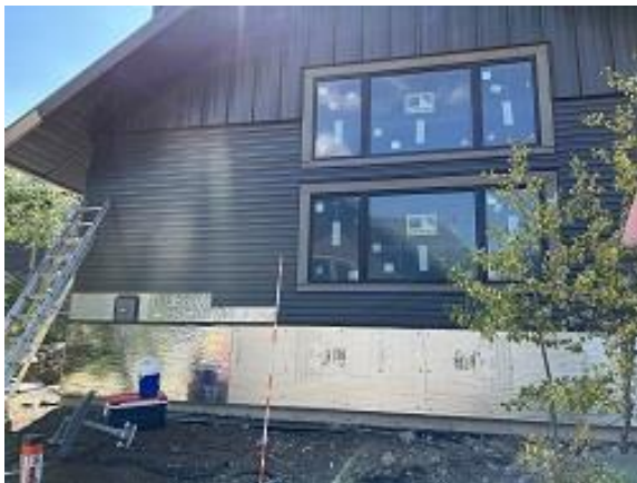
Building C2 Unit 14 Side Lap Siding Removed at Fireplace Vent
