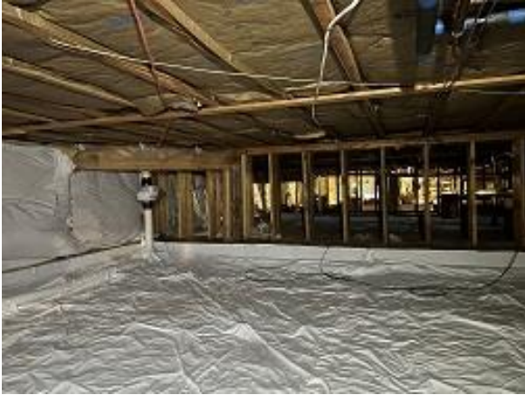
Building E1 Unit 9 Radon System Installed
