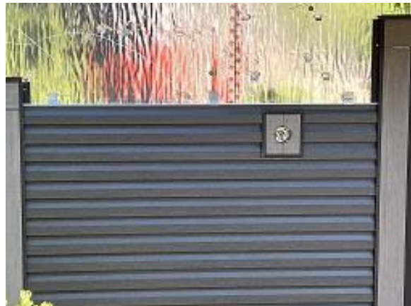
Building C2 Unit 14 Back Lap Siding Installed Clips More Than 24 Inches Apart
