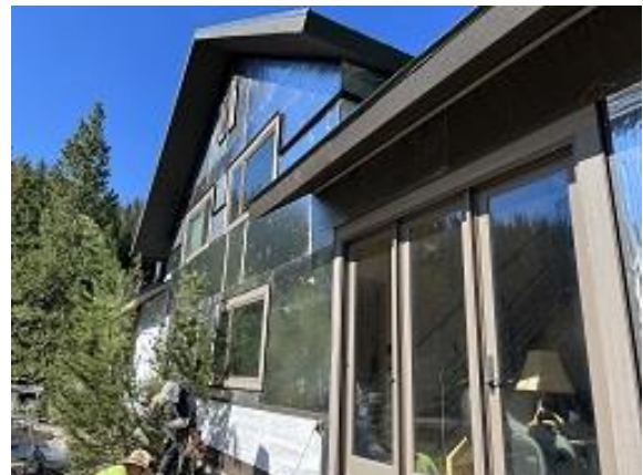
Back Window & Door Trim, Snap Batten Flashing, J Channel and Foam Board Installed
