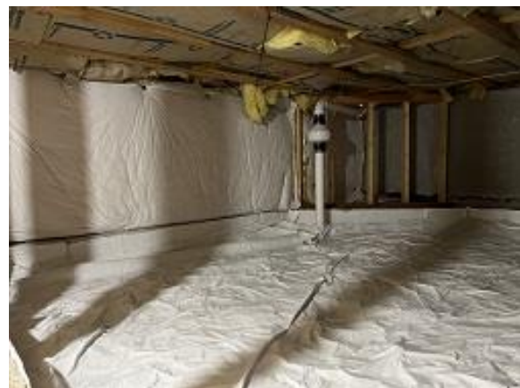
Building E4 Unit 30 Radon System Installed
