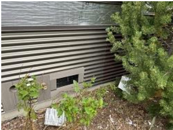
Building C7 Unit 59 Back Corrugated Siding Mismatched Color Installed
