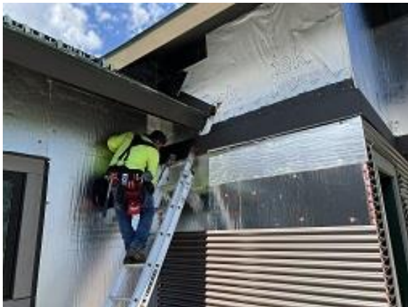
Building C7 Unit 60 Front Diverter Installed
