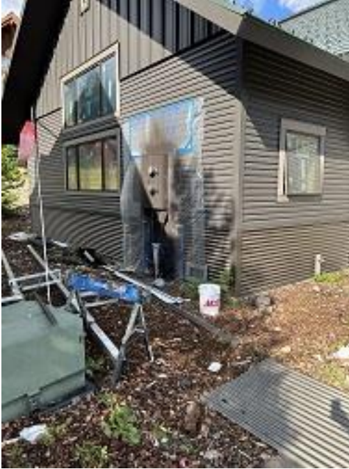
Building C8 Unit 66 Electric Panel Painted
