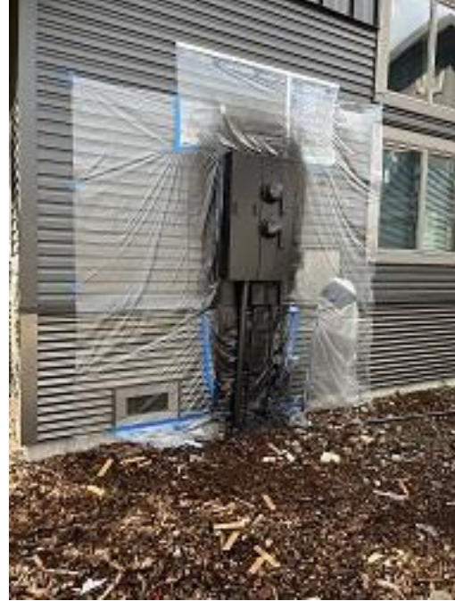
Building C9 Unit 67 Electric Panel Painted
