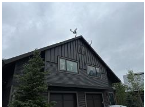
Building C7 Units 59 & 60 Satellite Dishes Installed
