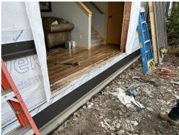
Building C10 Units 70 Deck Door Removed Mold on Threshold
