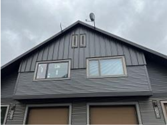
Building C9 Units 67 & 68 Satellite Dishes Installed
