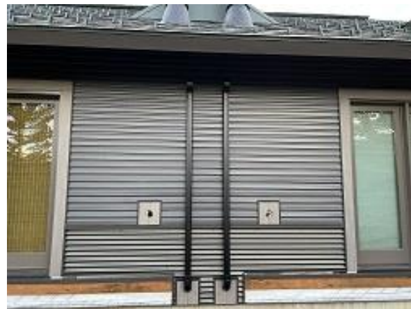
Building E8 Units 56 & 57 Back Radon System Vents
