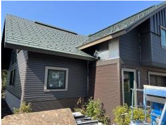
Building C6 Unit 54 Diverter Installed Appears Too Obtuse an Angle
