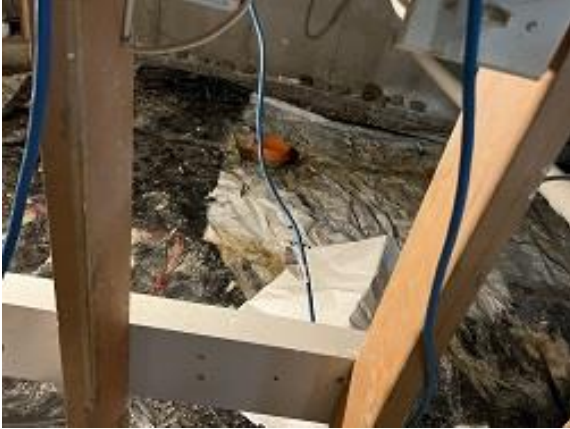
Building E9 Unit 62 Crawl Space Sump Pump Found During Radon System Install
