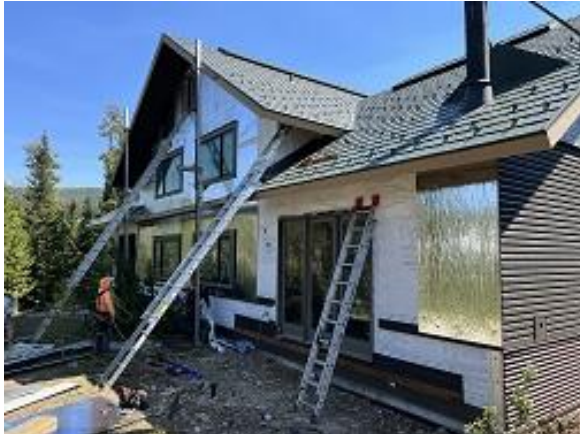
Building C6 Units 53 & 54 Back Foam Board Insulation, Window Trim & J Channel Installed
