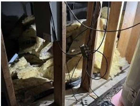
Building E9 Unit 61 Crawl Space Insulation Was Down Needed Moved for Radon System Install
