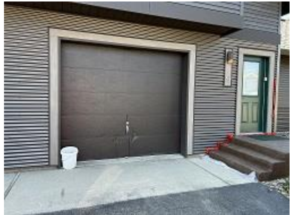
Building E1 Unit 9 Garage Door Damaged
