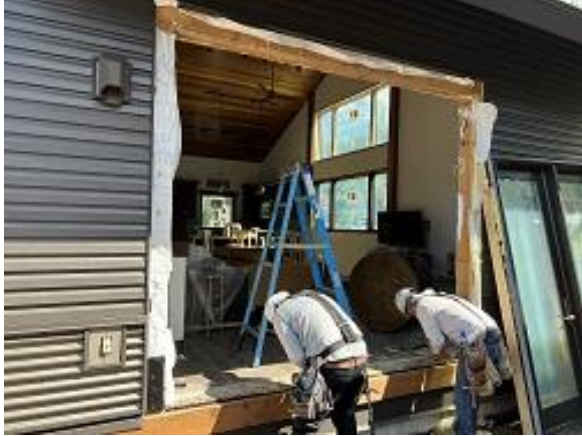
Building C5 Unit 39 Deck Door Removed to Correct Install
