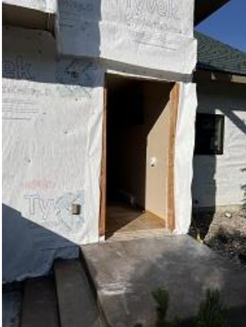
Building C4 Unit 35 Front Door Removed
