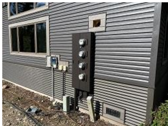
Building E8 Unit 58 Side Electric Panel Painted
