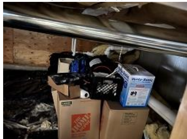
Building E9 Unit 61 Crawl Space Stored Items Needed Moved for Radon System Install
