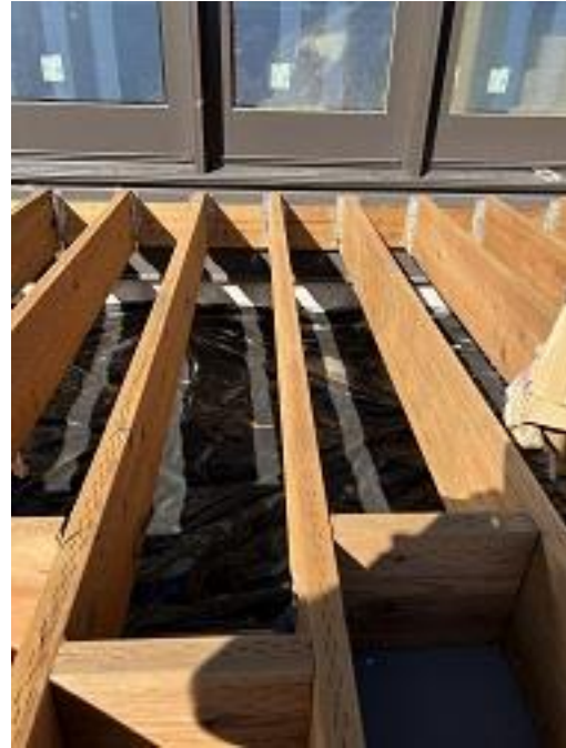
Building D Unit 37 Deck Framing Ledger Board Check Longer Than 3 in
