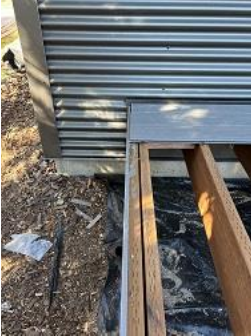
Building C3 Unit 32 Decking Inconsistent Cuts
