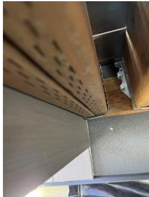
Building C9 Unit 68 Deck Ledger Missing Fasteners
