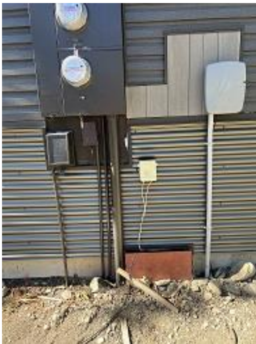
Building C1 Unit 12 Side Water Meter Attached to Siding
