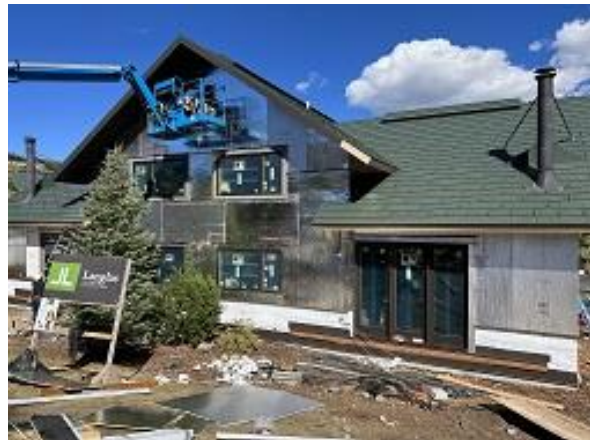
Building C4 Units 34 & 35 Back Head Flashing, Insulation Board, Window Trim & J Channel Installed
