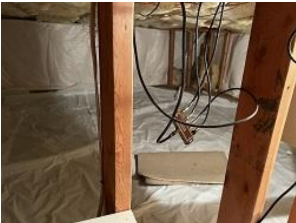
Building C9 Unit 68 Crawl Space Radon Existing Vapor Barrier Accepted
