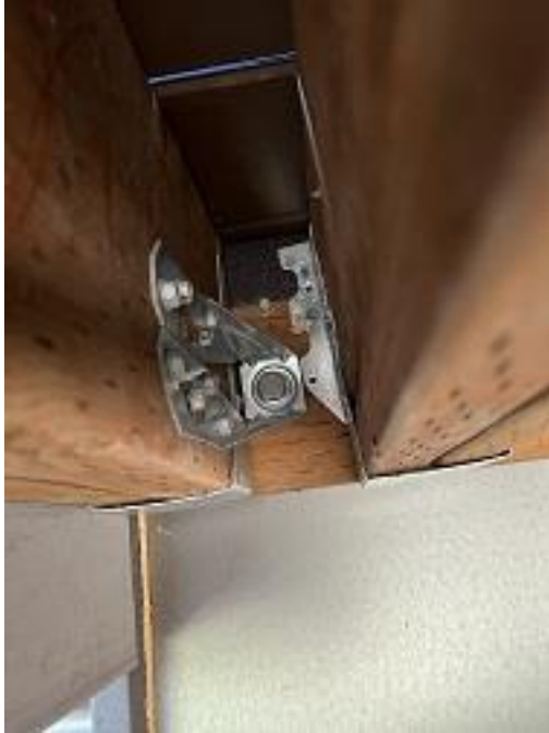
Building C6 Unit 53 Deck Ledger Wrong Fastener
