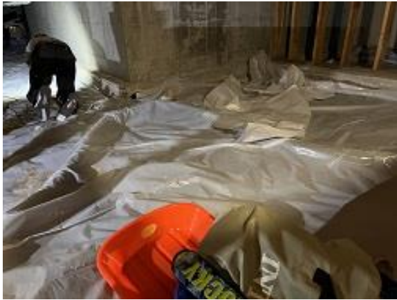
Building A Unit 2 Crawlspace Radon Remediation Damage Vapor Barrier Removed and Reinstalled
