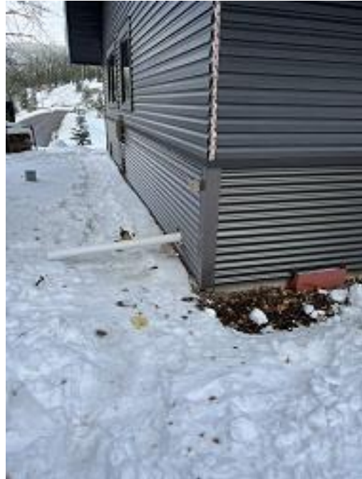
Building B Unit 7 Side Radon Exhaust Penetration
