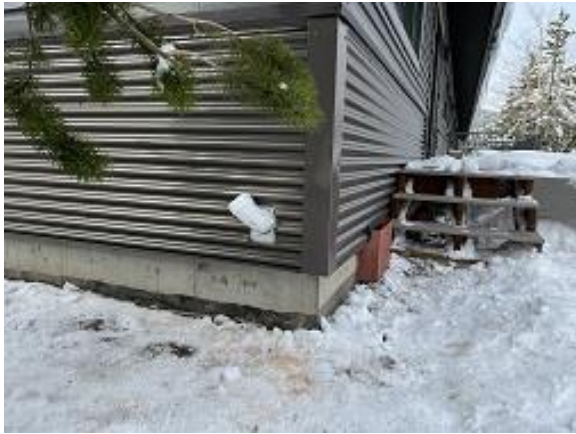
Building B Unit 3 Side Radon Exhaust Penetration
