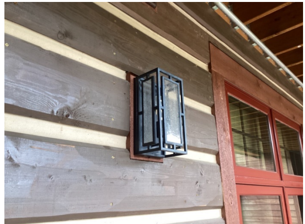
Building Two wall mounted light fixture
