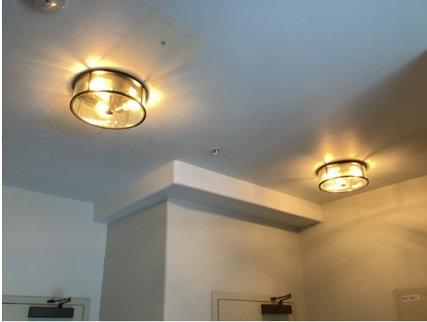
Elevator landing lighting
