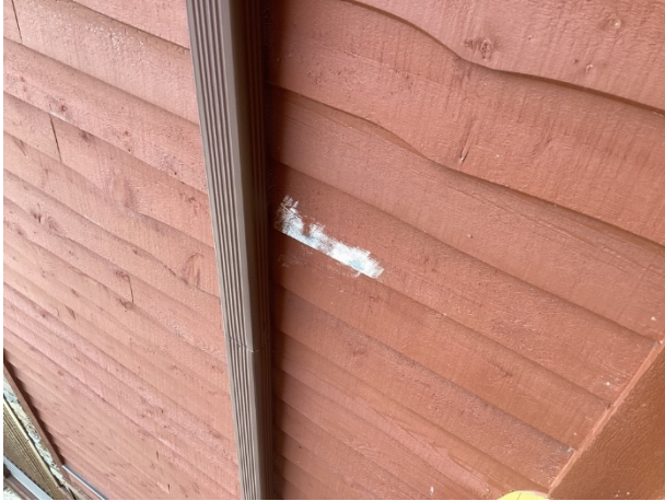
Siding finish loss near downspout at Building One
