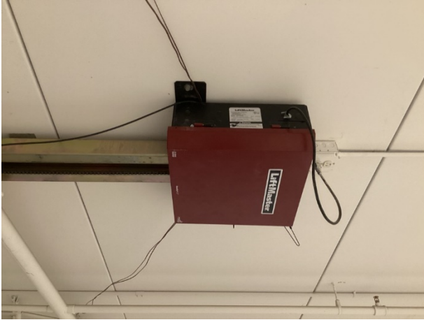
Garage door operator at Building Two
