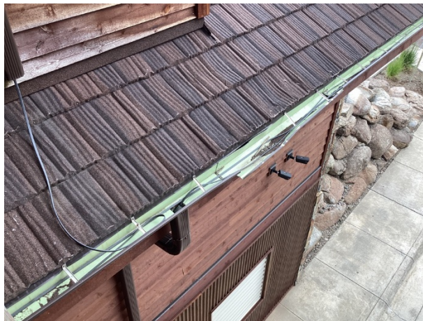
Gutter damage and heat tape at Building Two
