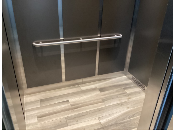
Elevator cab finishes at Building Two
