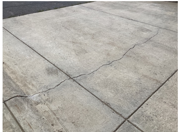
Cracks at Building Two ramp
