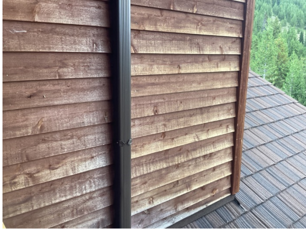
Finish wear at siding at Building Two
