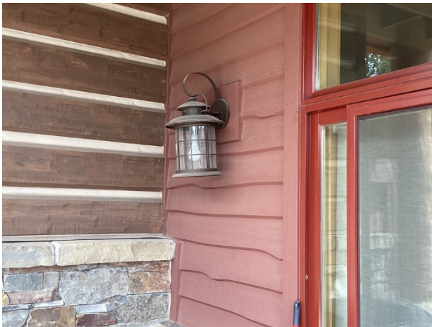
Building One wall mounted light fixture
