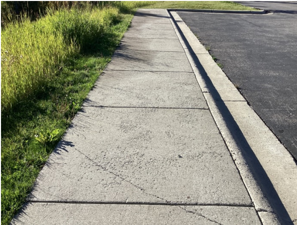
Sidewalk spalls and cracks
