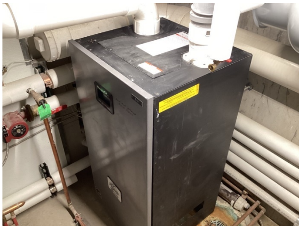
Boiler at Building Two
