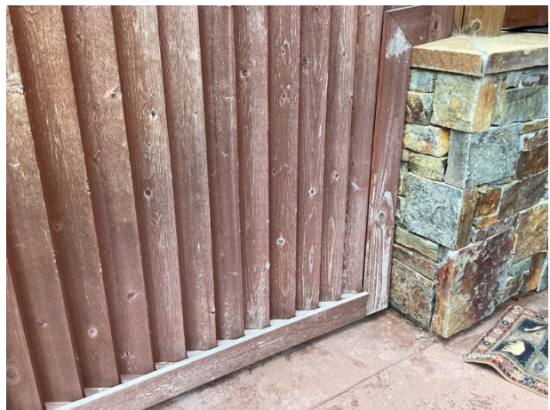
Privacy wall finish loss at Building Two
