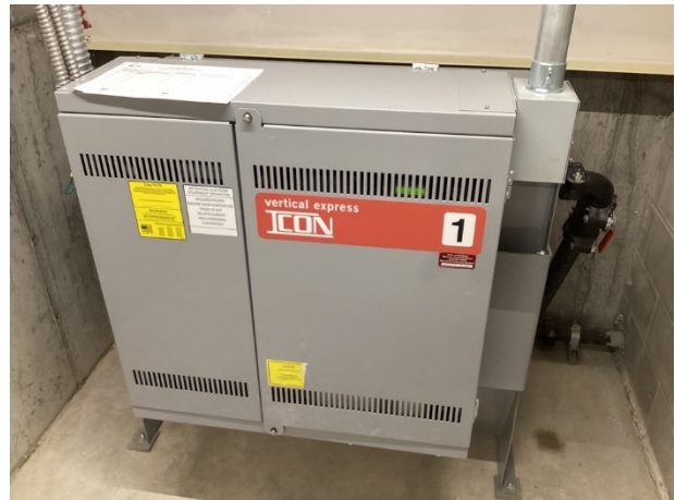
Hydraulic elevator equipment for Building Two
