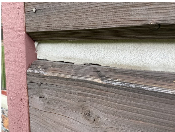
Isolated chinking deterioration
