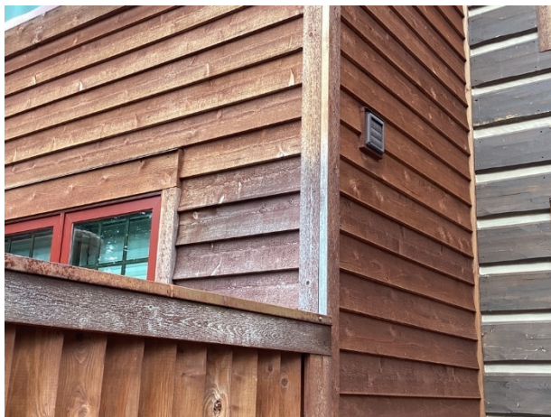
Finish wear at siding at Building Two
