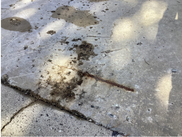
Exposed rebar at Building One entry sidewalk
