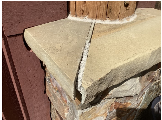
Capstone mortar loss
