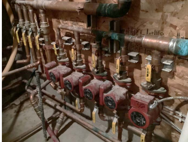
Building One circulation pumps
