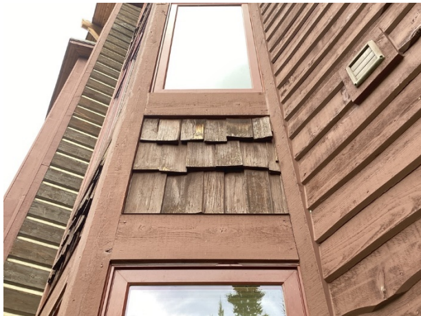
Finish deterioration at shake siding at Building One
