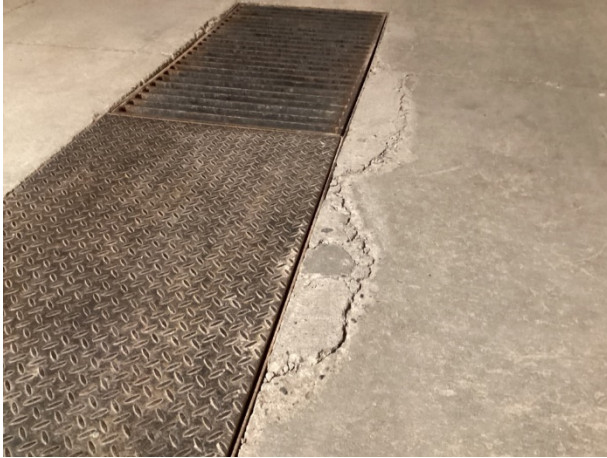
Cracks near drainage vault
