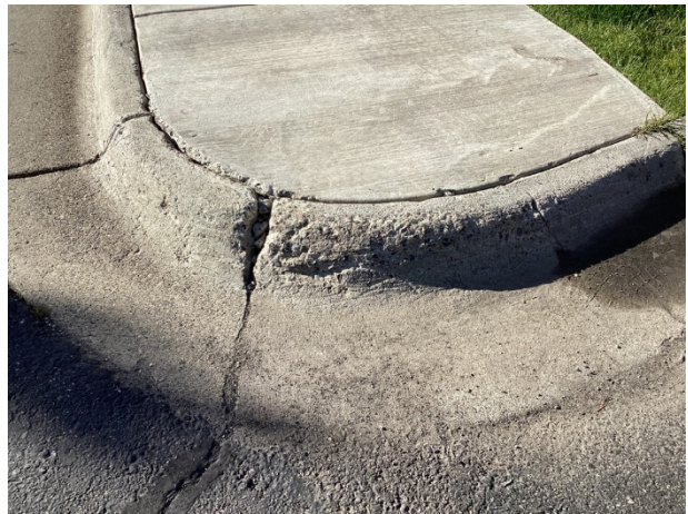
Curb spalls and cracks
