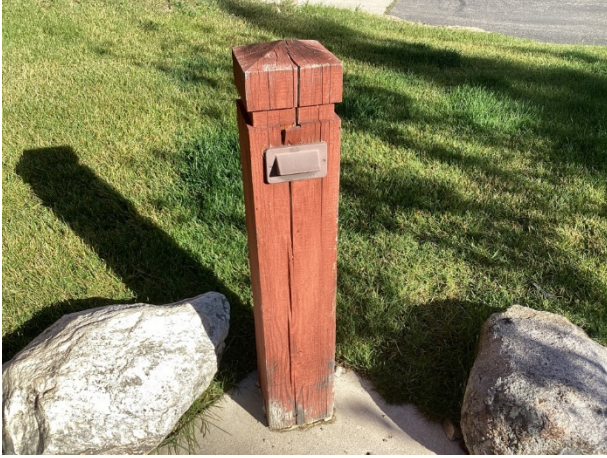
Bollard light fixture
