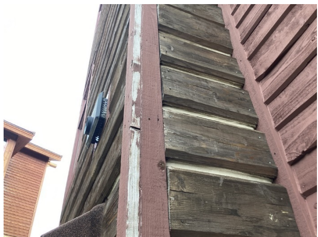
Corner trim finish wear at Building One
