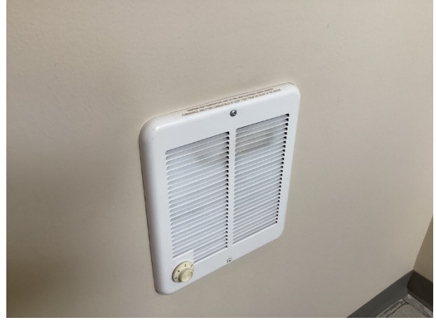
Stairwell unit heater
