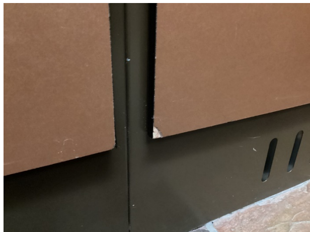
Wall damage at Building One
