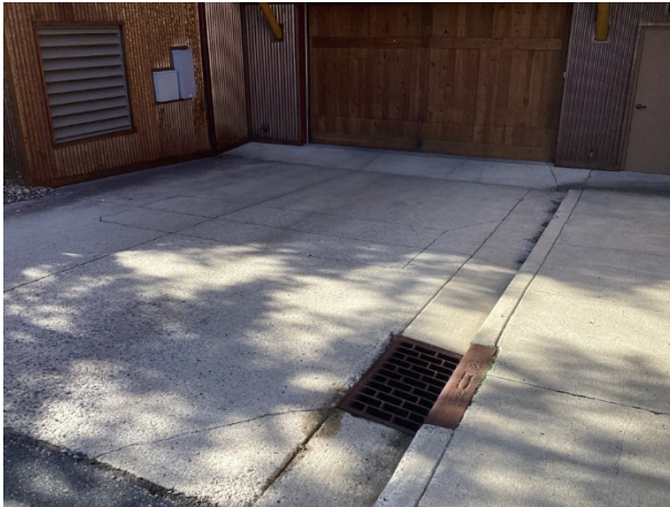
Garage ramp with snow melt system at Building One
