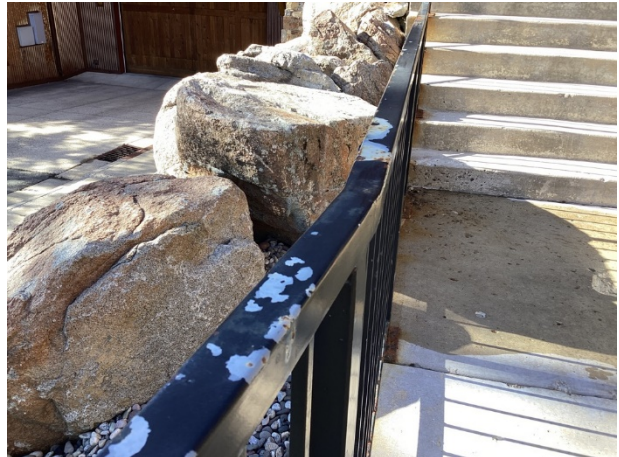
Railing finish deterioration
