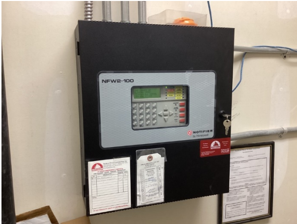
Control panel at Building One
