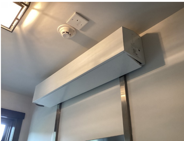
Building Two fire door
