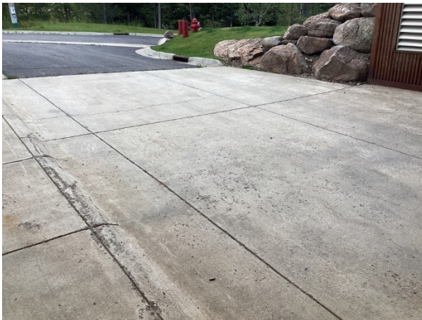
Garage ramp with snow melt system at Building Two
