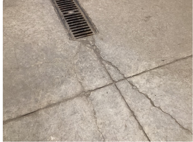
Cracks near drain
