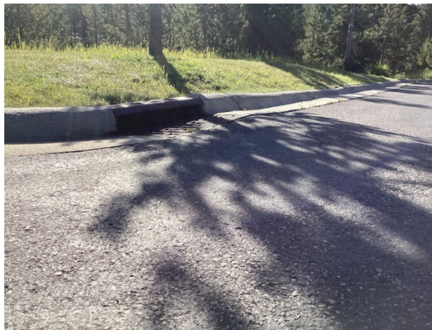
Heaves near catch basin
