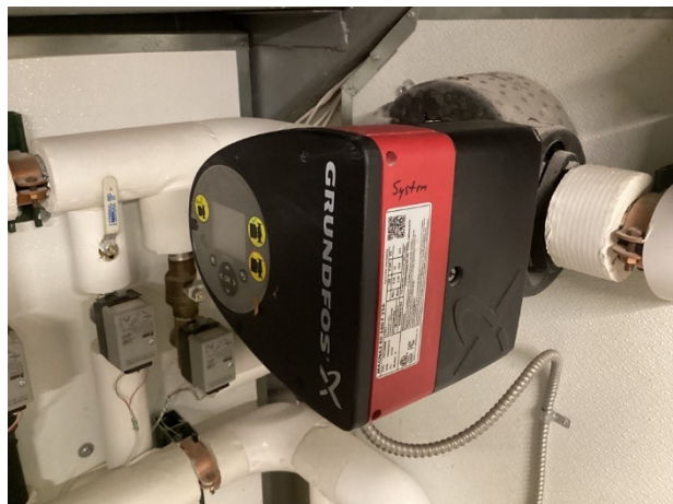
Building Two circulation pump
