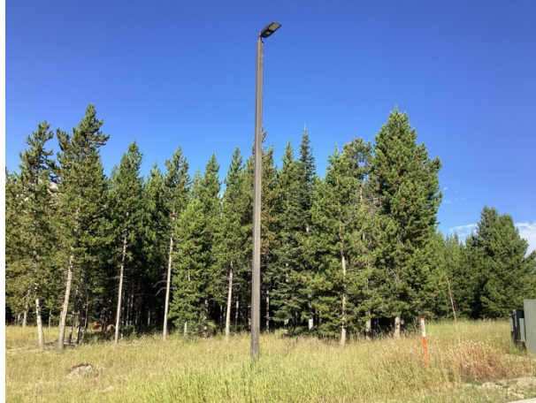
Light pole and fixture
