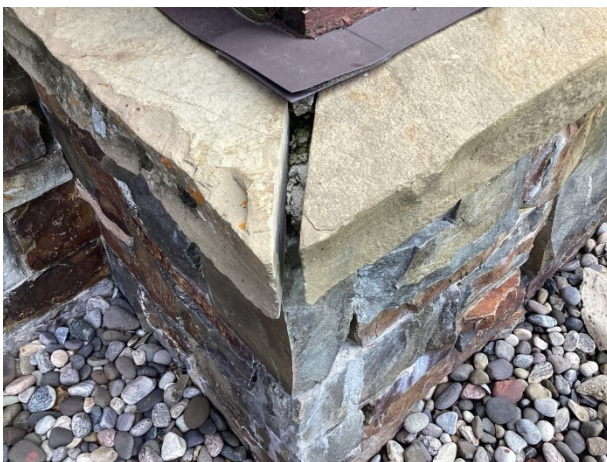
Sill mortar loss
