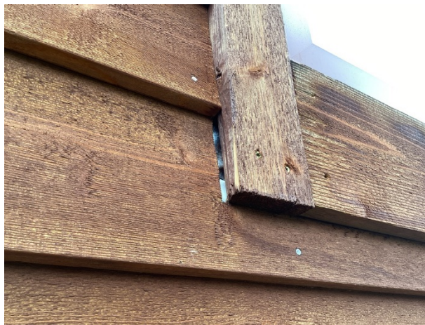
Gap between trim and siding at Building Two
