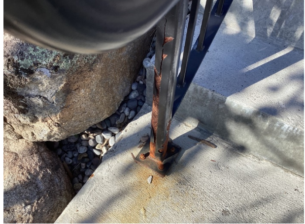
Building Two railing base rust
