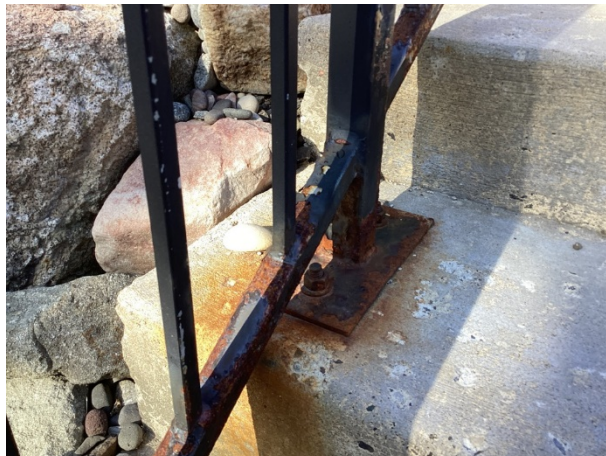
Significant base rust
