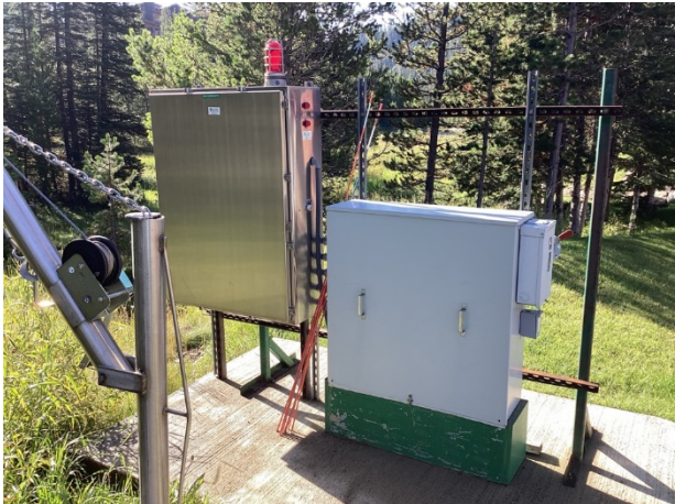
Lift station controls
