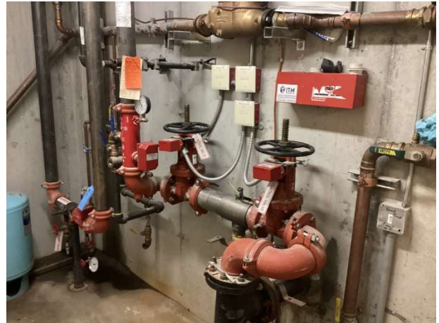
Large diameter valves
