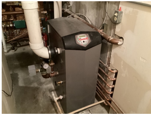
Boiler for snow melt system, garage and elevator landing heating for Building One
