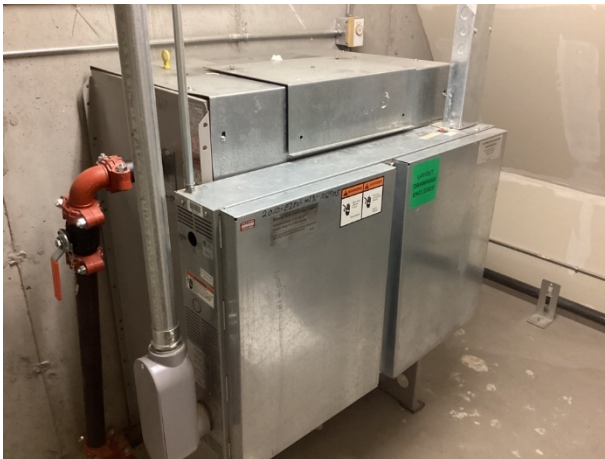
Hydraulic elevator equipment at Building One
