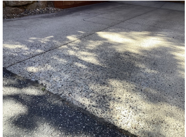
Building One ramp spalls
