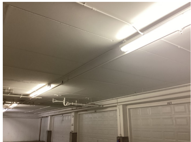
Garage light fixtures
