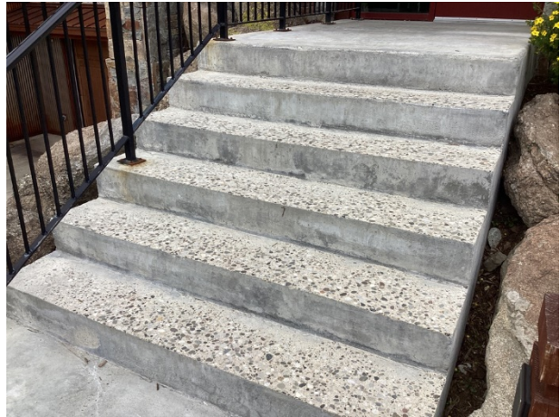
Building Two previous grinding repairs
