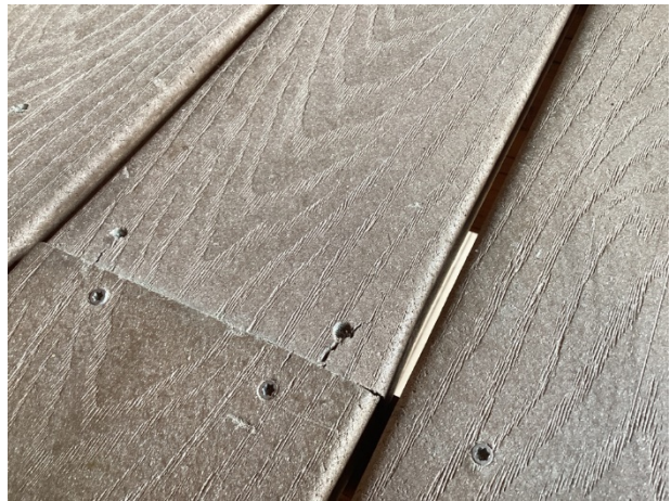
Decking cracks at fasteners
