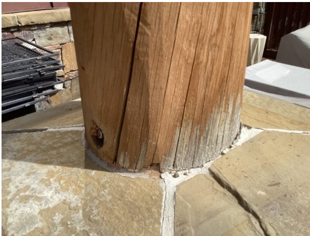
Timber balcony post base weathering
