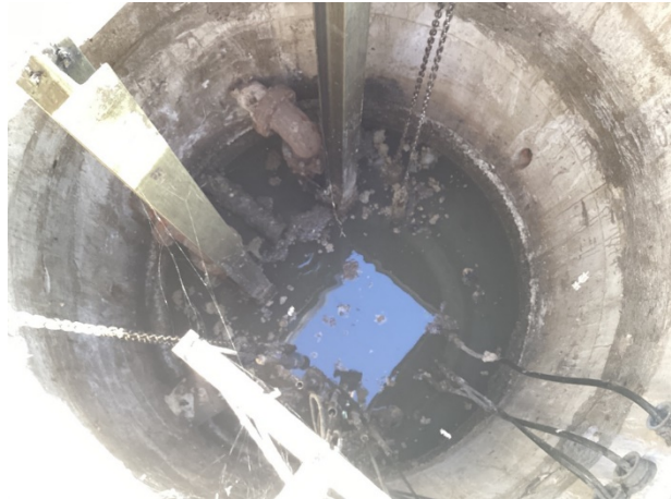
Lift station pumps
