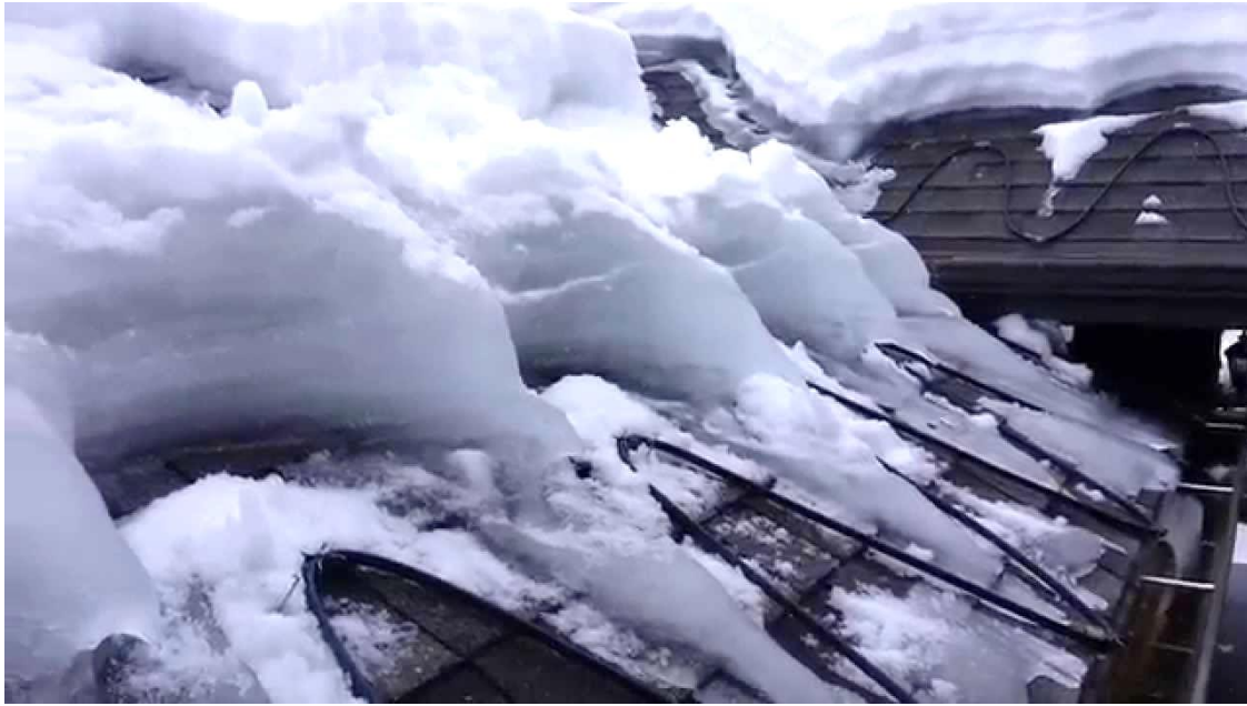
Heat tape tends to migrate the ice dams and can often exacerbate the roof ice
