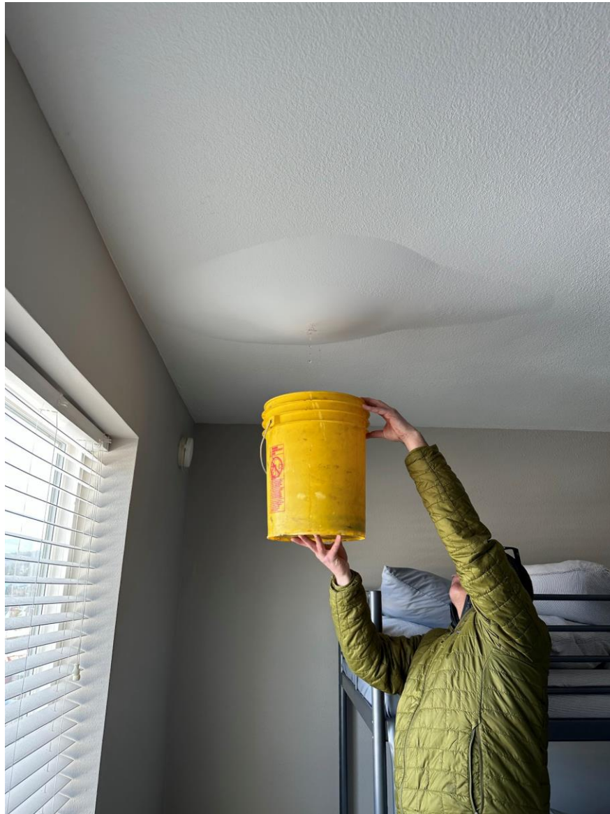
A roof leak is penetrating a bedroom in condo building C
