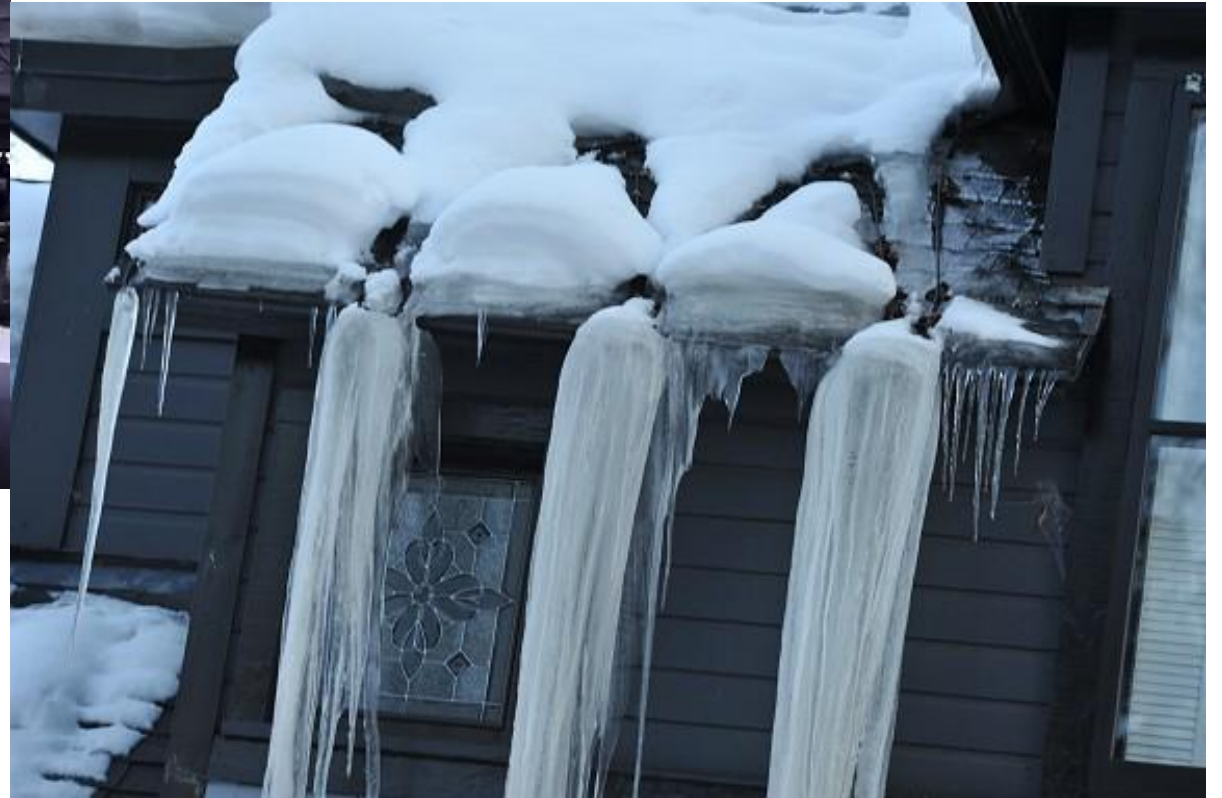
Icicles from heat tape damage siding and create dangerous safety conditions
