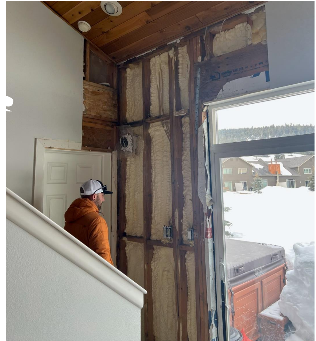
This roof leak and remediation displaced the owners for approximately 3 months
