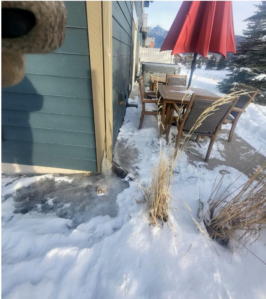
Roof heat loss and ice formation damages gutters, siding, and creates unsafe conditions on ground level
