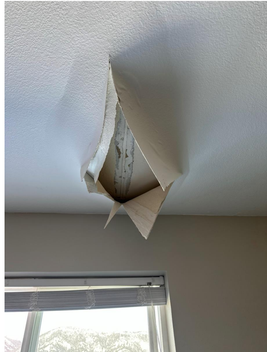
This type of drywall damage is common throughout the association due to roof leaks
